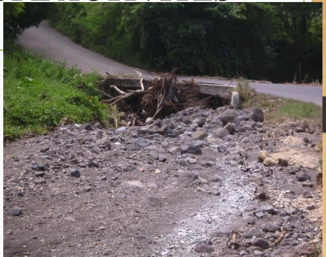
Rock slides blocking drains in Folly Ghaut Valley
